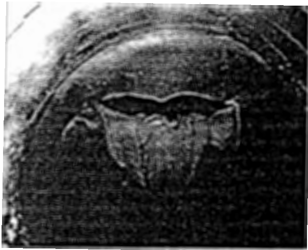
Figure 13.6 Collapsed scotch marine boiler's corrugated furnace caused by scale and dry firing. (Courtesy Royal Insurance Co.)
